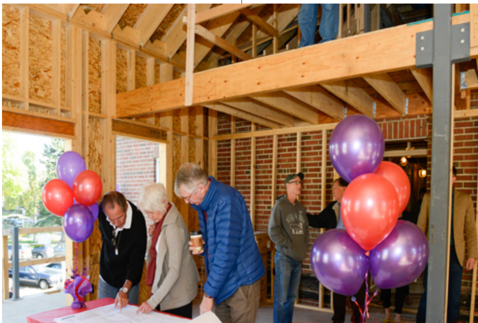
Brothers tour the progress of construction in the new library during the Centennial Anniversary Celebration.
